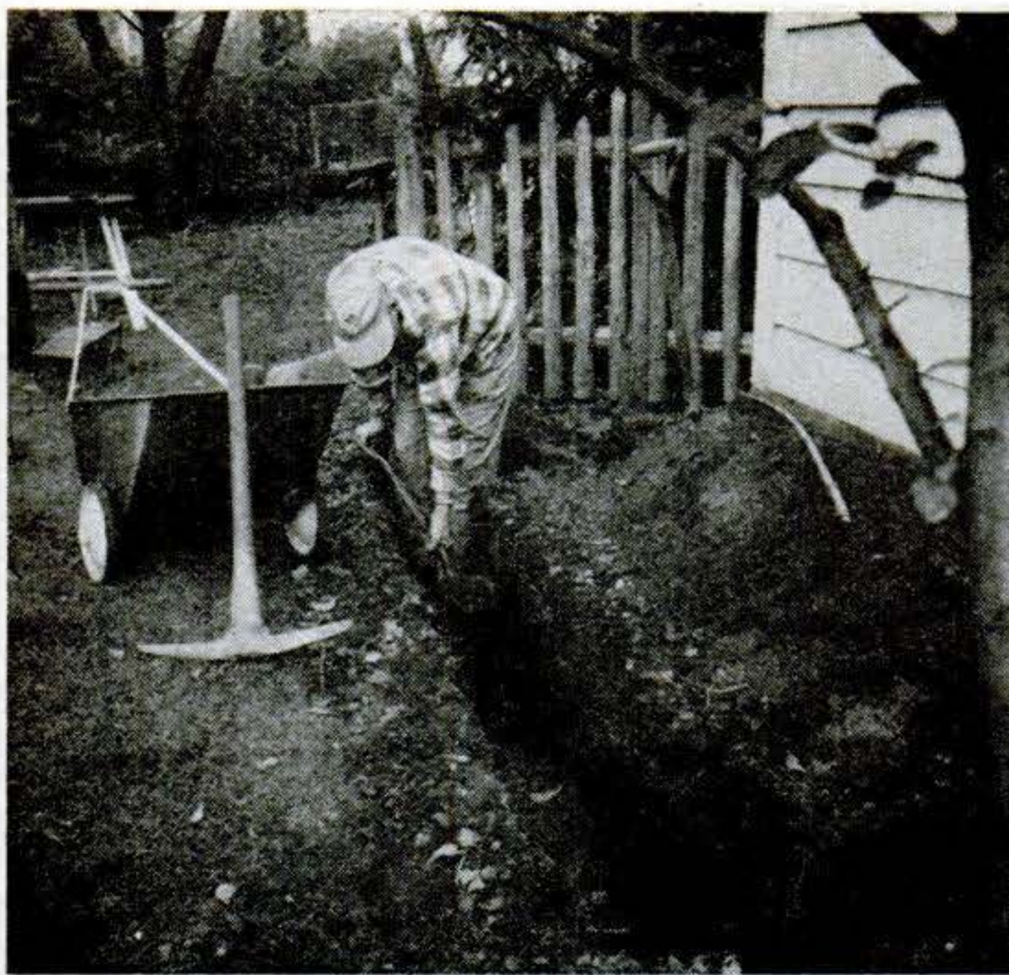
1 FOUNDATION TRENCH outlines the new extension. Dig it below frost line and about a foot wide. Pour in concrete footing and level it off 20" below the ground.
